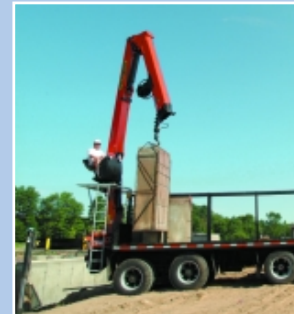
A high inner hook height allows the crane to reach and lift the 1st cage with ease
